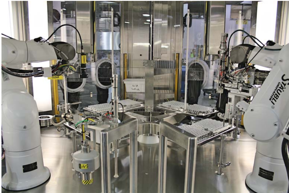
Figure 3 - AseptiCell robotic aseptic filling system utilizes two vision guided Staubli Stericlean or HE robots (courtesy of Automated Systems of Tacoma, Inc.)
