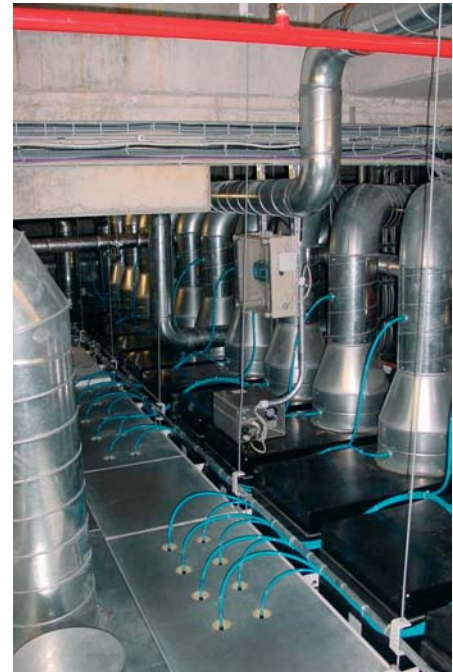
Infrastruktur zur Partikelmessung. Blick hinter die Decke. Infrastructure for particle measurement. A glimpse behind the scenes
